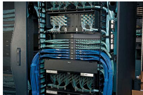
Figure 6. PANDUIT® QUICKNET™ Angled Modular Patch Panels and Cabling Assemblies reduce deployment times and optimize space in dense patching environments.
