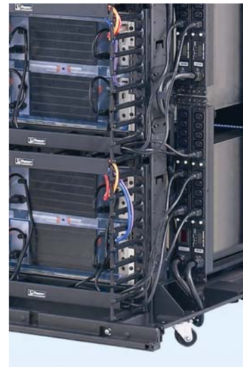
Figure 5. POU mounting locations help keep air exhaust pathways behind servers clear to provide maximum airflow and enhance equipment cooling.
